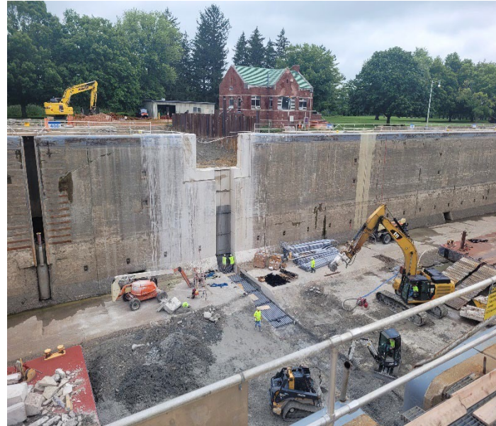
Marseilles Electrical Crossover
