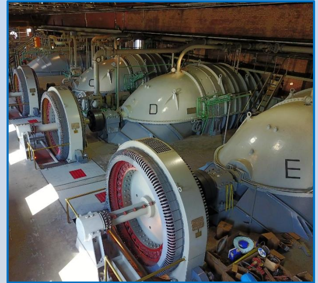
Drainage Pumps with 25 Hz Motors
