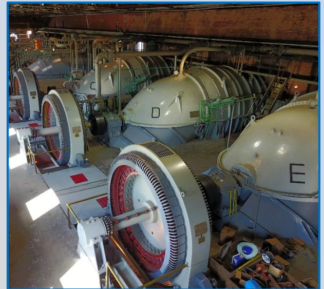
Drainage Pumps with 25 Hz Motors
