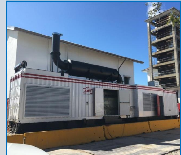
EMD 25 Hz Generator
