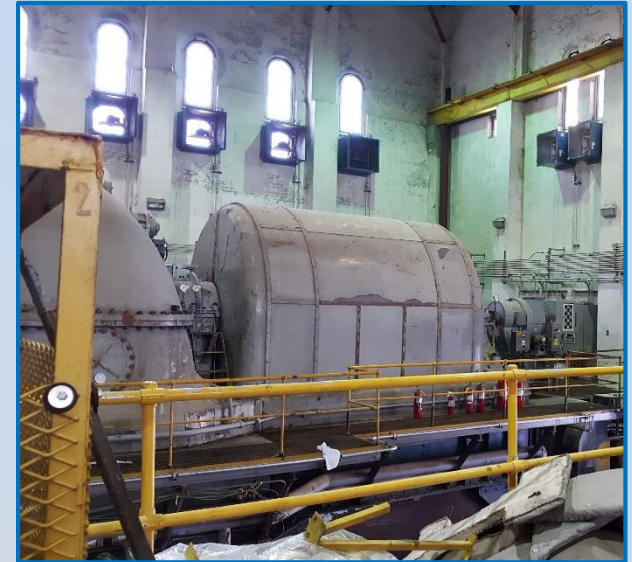
25 Hz Turbine Generator (20 MW)
