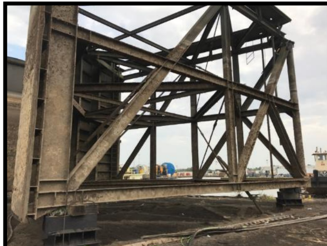
West Gates removed from Lock prepped for steel repair, sandblasting and painting
