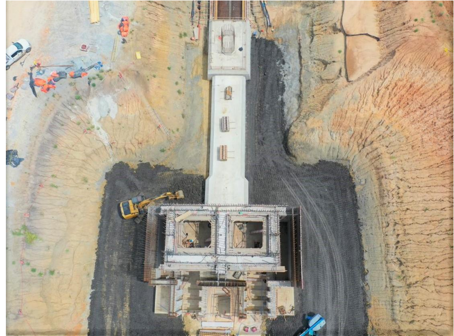
Two 78-inch pipes carry water from the Intake Tower to Raw Water Pump Station
